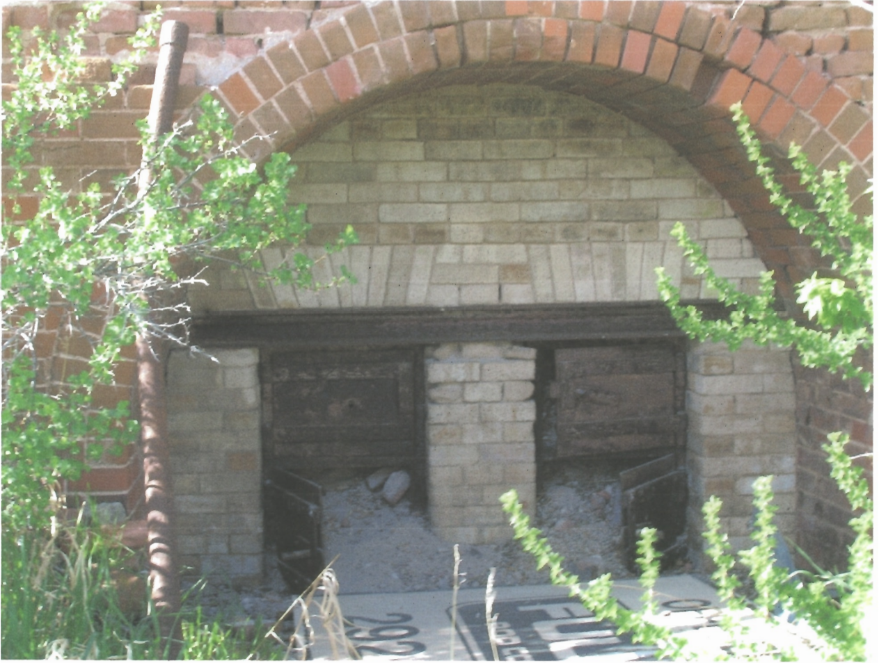
13. Remains of the Silica lime kiln at the site of the Silicated Brick Company- May, 2006 Close-up view of the doors.
